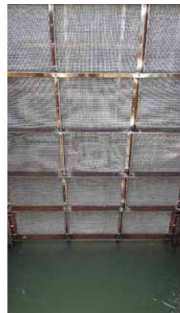
Band screen installed and water level is transmitted by ultrasonic water level sensor.
